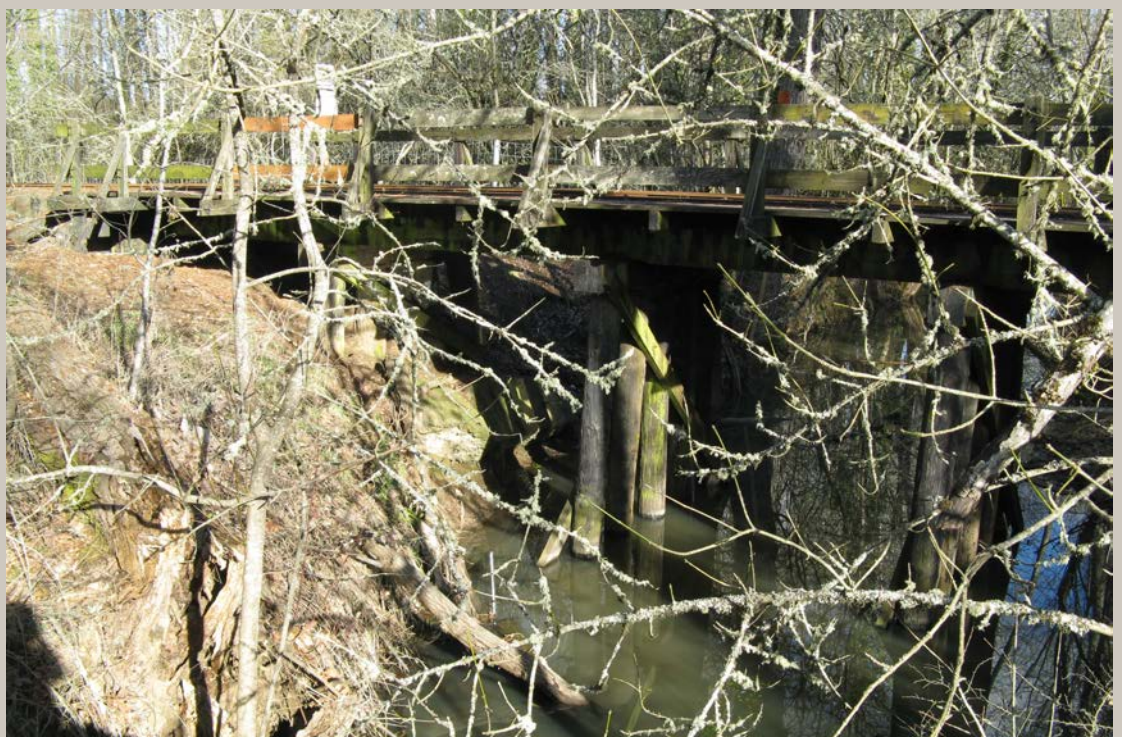
At Marysville Golf Course south of Avery Park, an old railroad trestle crosses the Mill Race. (Photos: Lee Sherman)
